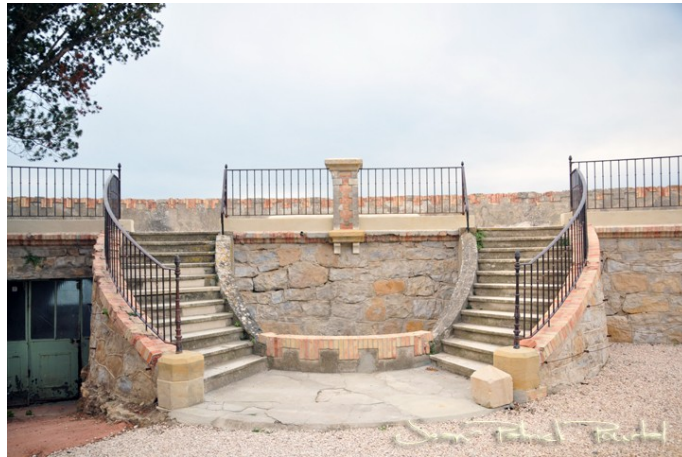
Part of "Belvedere" between Tour Magdala and Orangerie: the double-winged escalier / stairway
